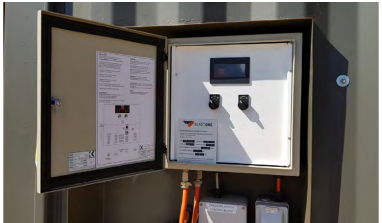
CONTROL CUBICLE WITH SWITCHES BEHIND WEATHER PROTECTION DOOR
