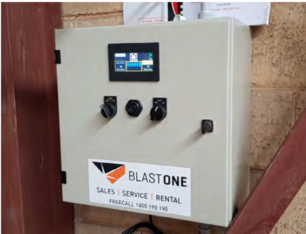
CONTROL CUBICLE WITH EXTERNAL SWITCHES
